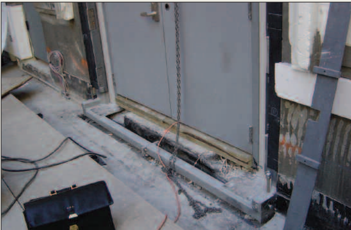
A special frame was embedded in the floor, walls, and ceiling to ensure that the doors would open and close flawlessly, with no vibration or space gaps. The floor piece had to be a perfect 90 degrees, and getting the entire frame precisely aligned was one of the greatest challenges of the job.
