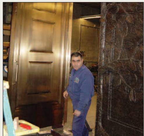
BOTTOM: The doors were assembled in the shop prior to final installation. The inner panels are a piece of art themselves, and are clad with muntz metal sheets, given a satin finish, and oxidized in a light brown.
